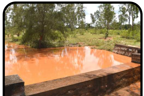
Rain water conserved in check dam at Kasthur
